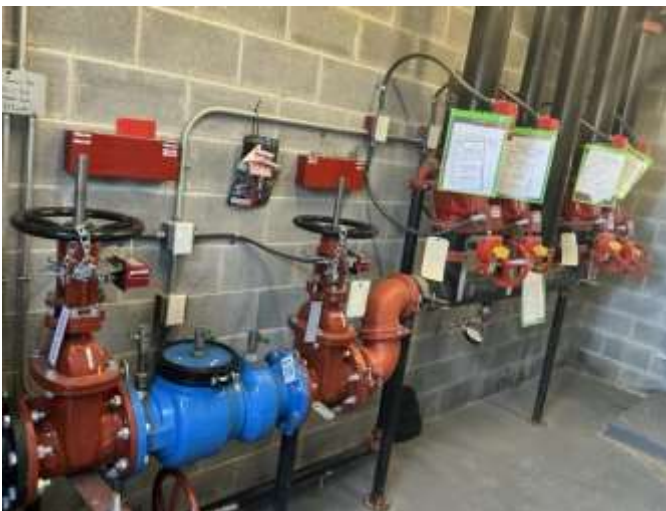
23 - FIRE SUPPRESSION SYSTEM
