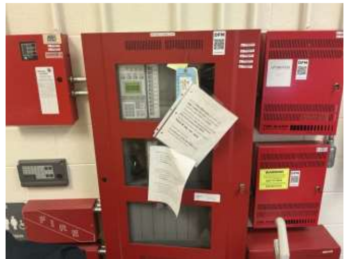
24 - FIRE ALARM PANEL
